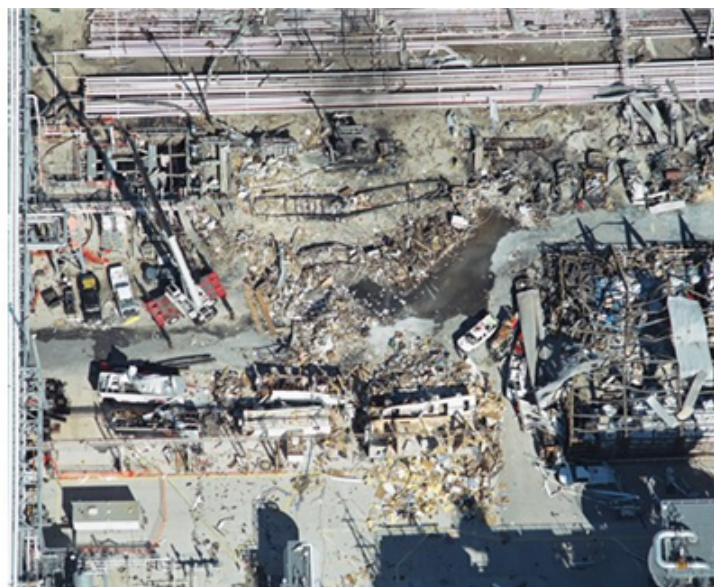
Figure 1: Aerial View of Damaged Buildings Caused by the Explosion 3
